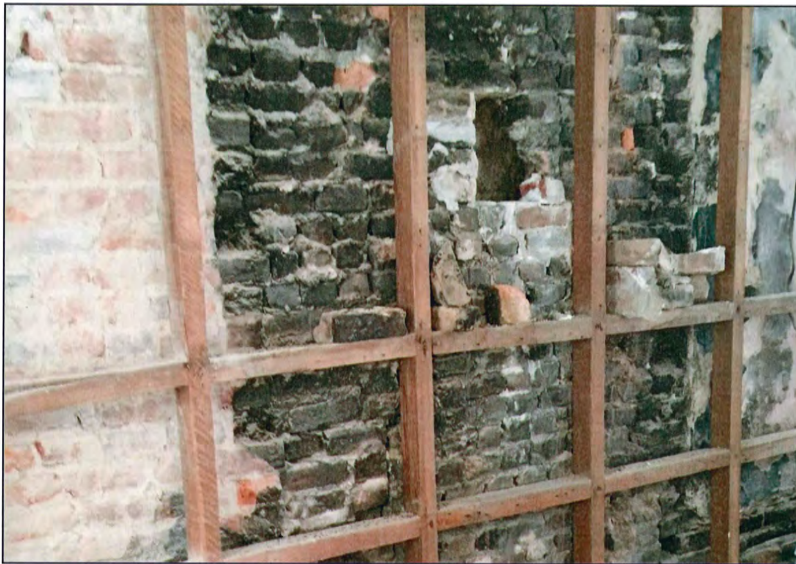
Figure 3: Voids in wall at chimney area. Fire damage to inset timbers.
