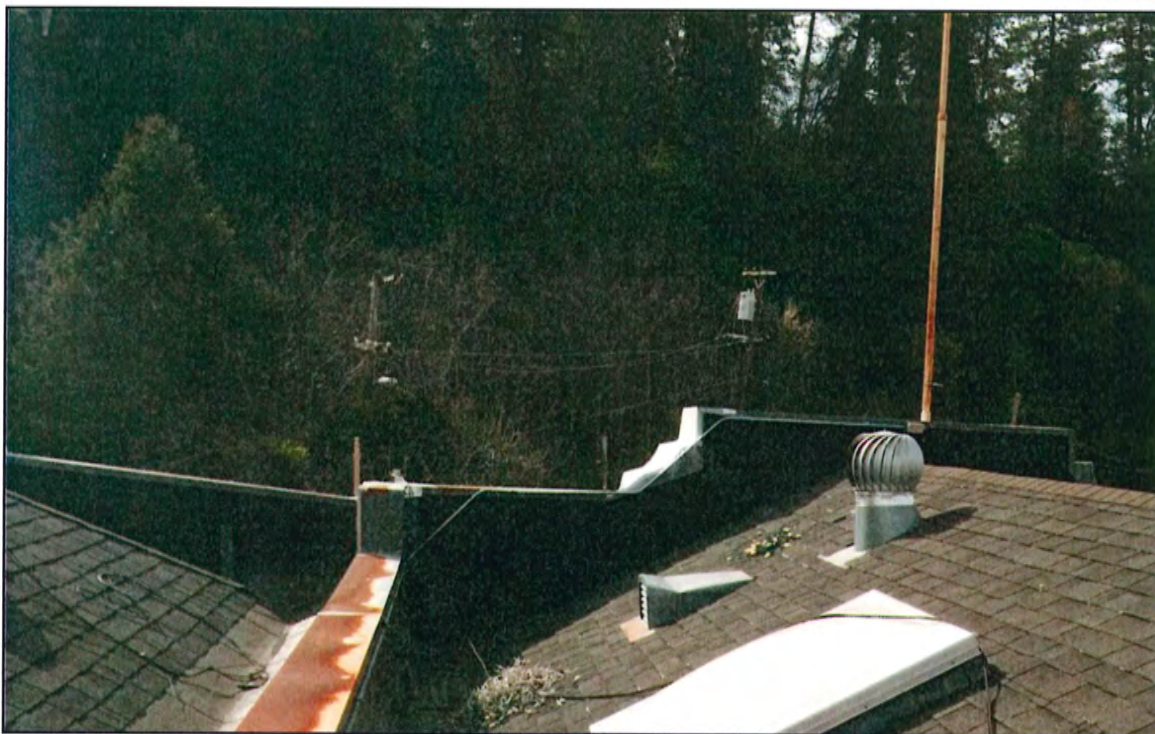
Figure 5: Unbraced roof parapet
