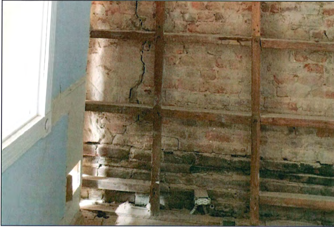
Figure 2: Deteriorated bed and head joints in masonry walls.
