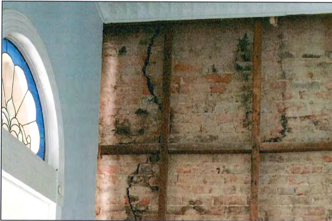
Figure 1: Large cracks in the west masonry wall.
