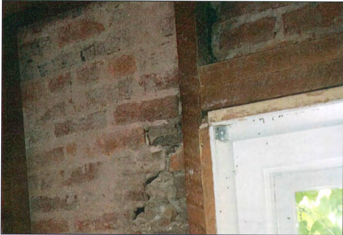
Figure 4: Door opening not integrated with lintel. Lintel to be reconstructed.
